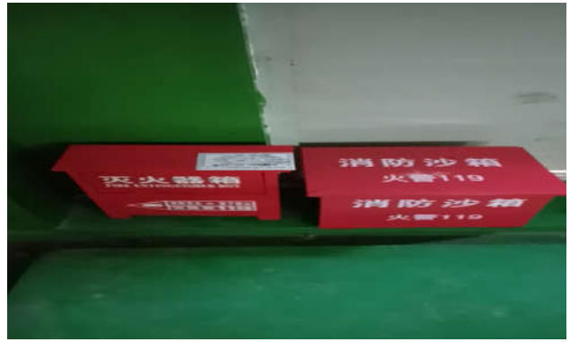
灭火器和消防沙箱
